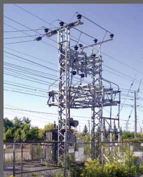
Before system upgrade
